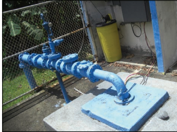
Figure 1. One of ASPA's 53 ground water wells. Wells are encased in concrete and may be as deep as 300 ft (90 m), requiring pumps of 30 to 40 hp (22 to 30 kW) to draw water to the surface. A 6% solution of sodium hypochlorite in the yellow drum is injected into the distribution system to disinfect the ground water as it reaches the surface.
